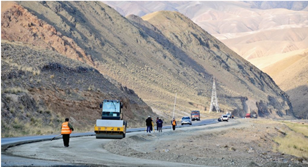
Mountain road construction. Workers are rehabilitating a road in the Kyrgyz Republic (photo by Asian Development Bank).
